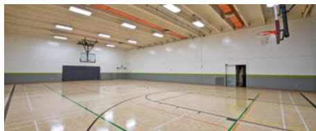
More than 3,320 lighting fixtures were upgraded to T-8 electronic fluorescent lighting throughout the 4 campuses saving 778, 100 kWh in electricity annually with no change in light levels.
